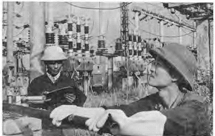
The An Lac transformer station in Haiphong heavily damaged by U.S. aircraft during the air war of destruction in 1972 has been repaired and is enlarging.
